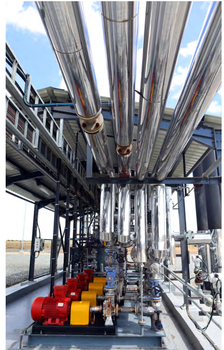
Conduction oil pumps.
