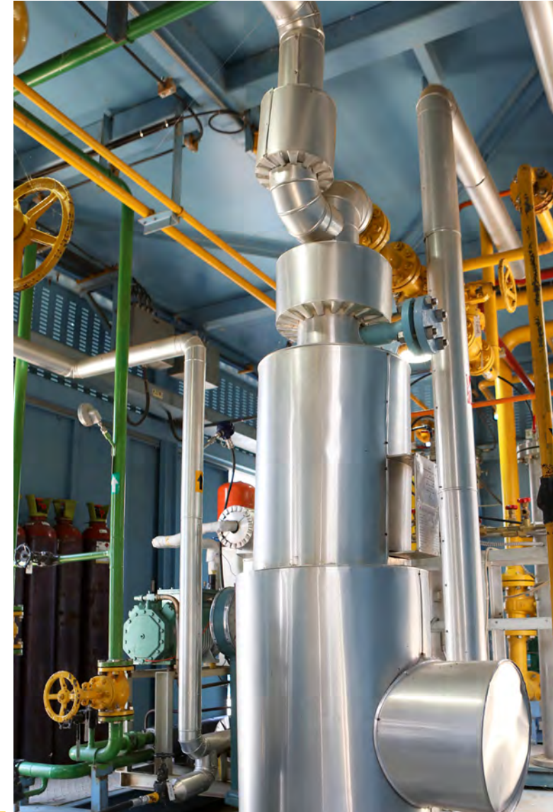
Mixed refrigerant loading manifold.
