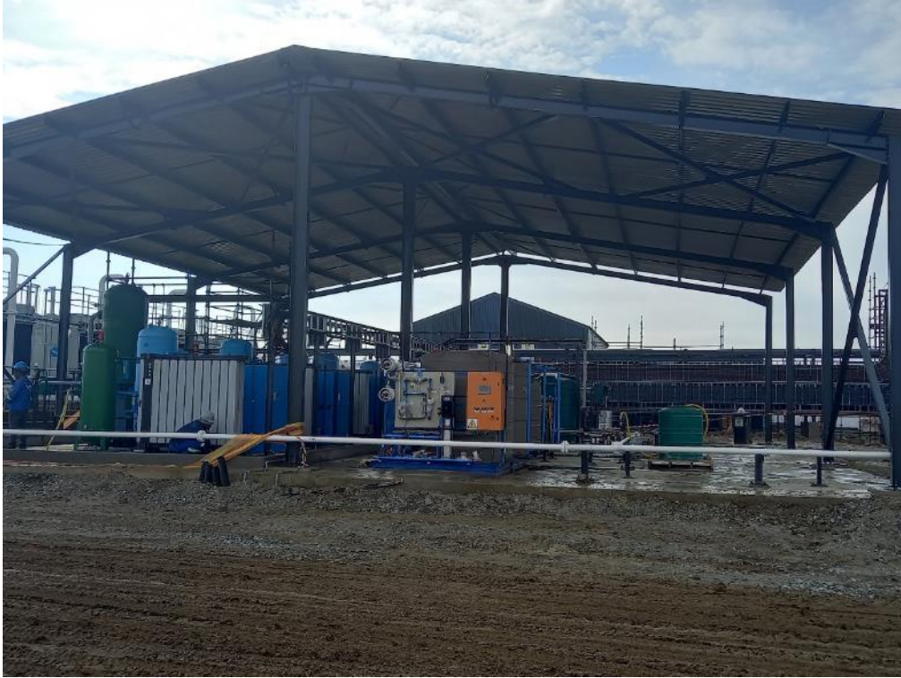
Figure 10: A roof was placed over the process water treatment plant at the BOP.
